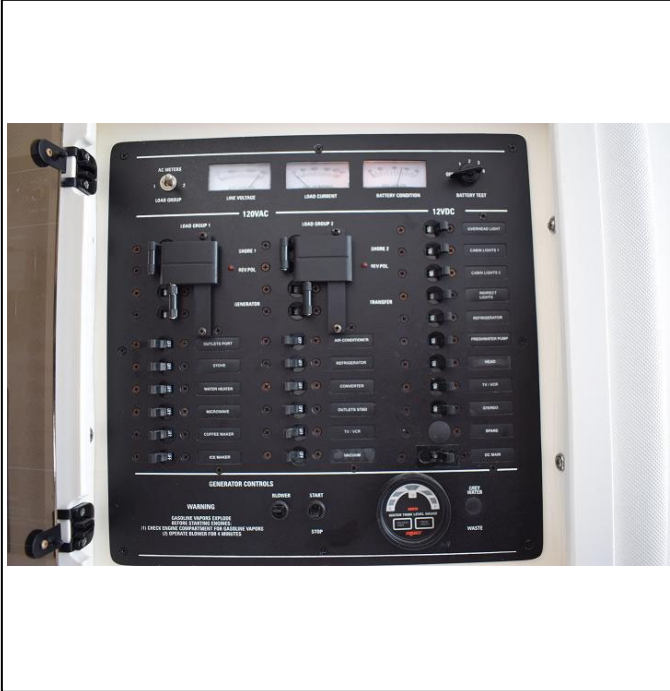
Main Electrical Panel
